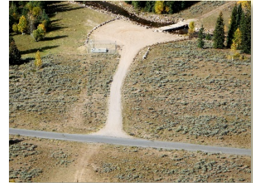
Existing North Fork Siphon Blow Off Structure with existing river crossing in the background
