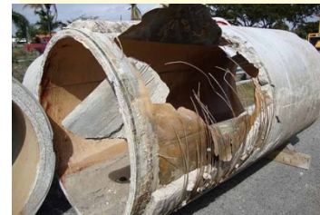
Failed PCCP in Miami, FL
