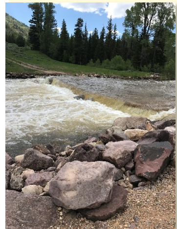
Overtopping of the North Fork of the Duchesne River Crossing
