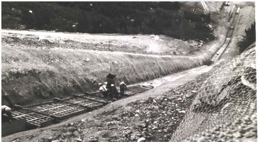
Contractor laying bedding material for the North Fork Siphon on the west slope.
