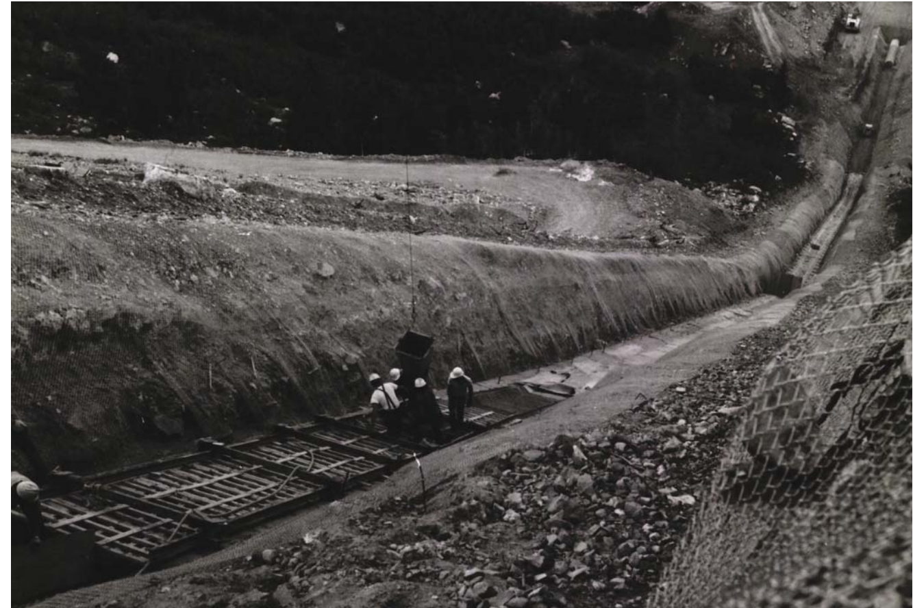
Contractor laying bedding material for the North Fork Siphon on the west slope
