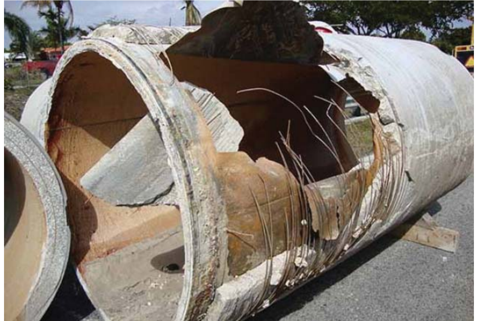
Failed PCCP segment in Miami, Florida
